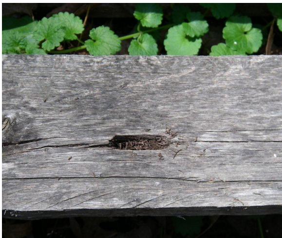
Section of a pallet showing tunneling and frass
